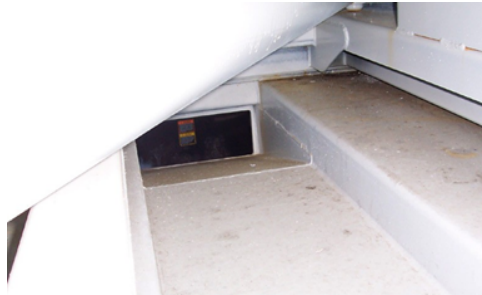
Figure 89. Inside Sump Door
