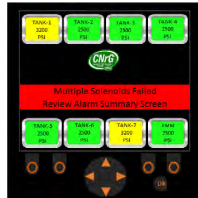
Figure 90. Display Screenshot: Multiple Solenoids Failed
