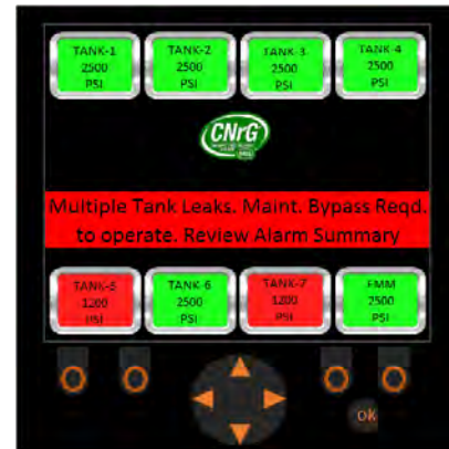
Figure 87. Multiple Tank Leaks. Maintenance Bypass Required.
