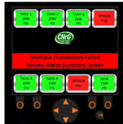
Figure 83. Multiple Pressure Transducer Sensors Unplugged/Faulty
