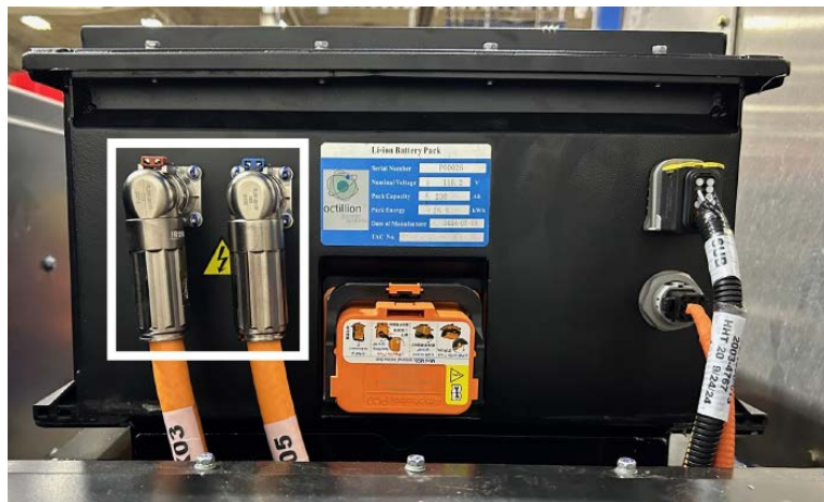
Figure 31. Battery High Voltage Power Connectors
