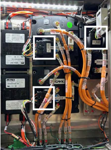
Figure 32. Body High Voltage Electrical Cabinet Panel 1 (3 Locations)
