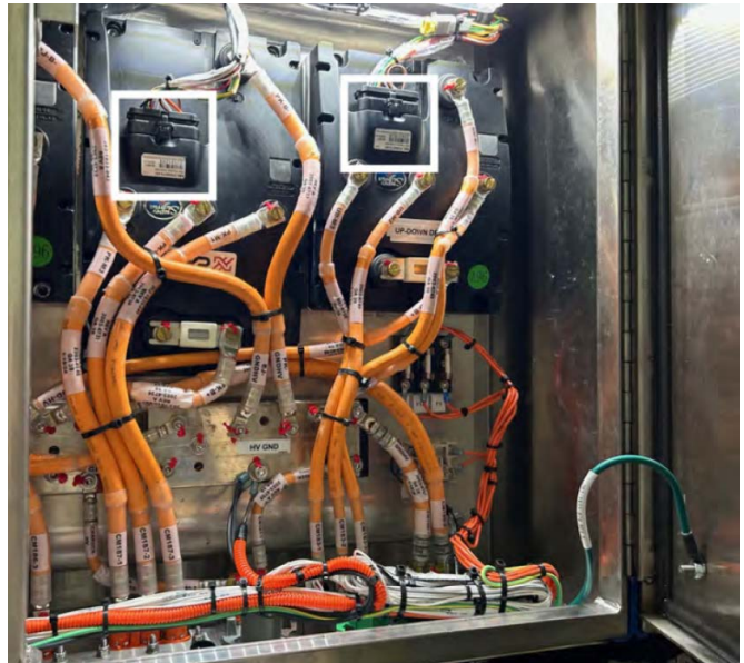
Figure 39. High Voltage Electrical Cabinet Panel 2 (2 Locations)
