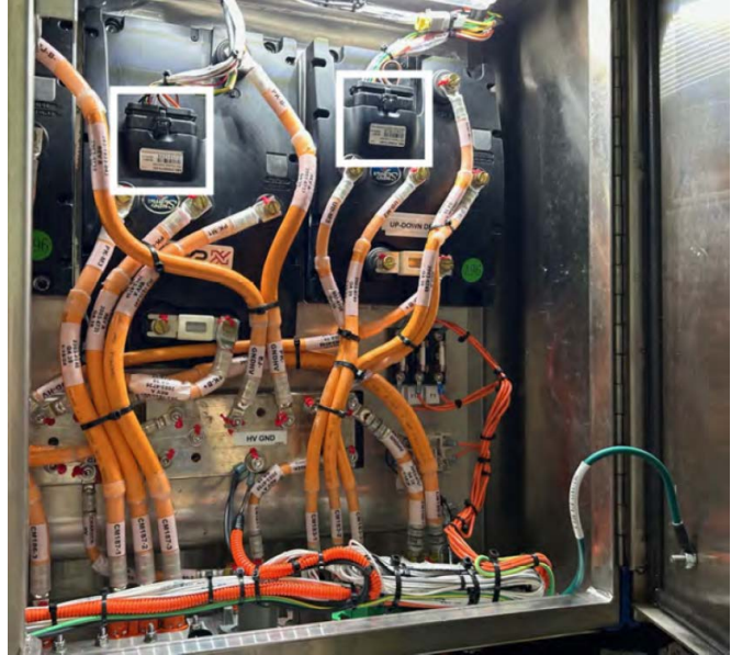
Figure 33. High Voltage Electrical Cabinet Panel 2 (2 Locations)
