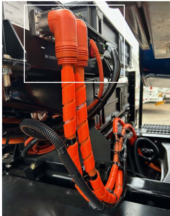
Figure 34. Location of the Battery Management System (BMS) Connectors
