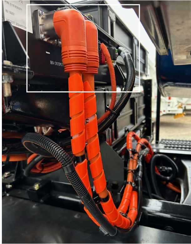
Figure 37. Location of the Battery Management System (BMS) Connectors
