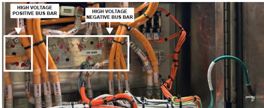
Figure 48. Body High Voltage Electrical Cabinet Panel 2 Voltage Testing Locations
