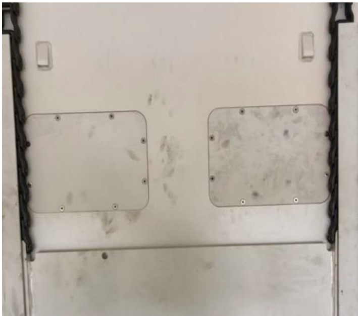
Figure 98. Closed Access Doors
