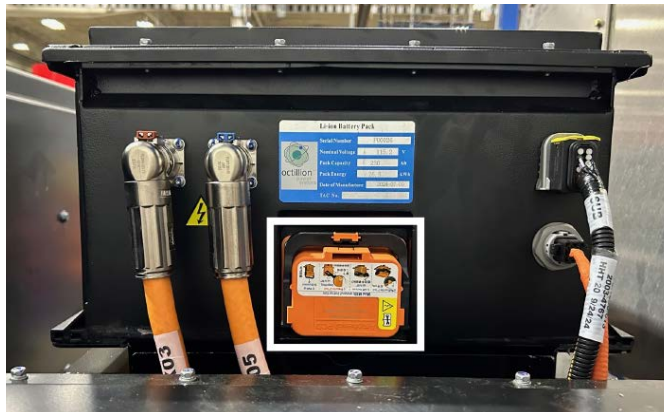
Figure 46. Main System Disconnect
