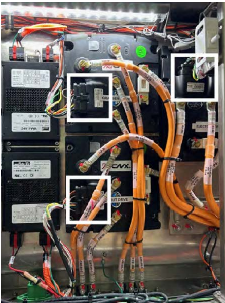
Figure 38. Body High Voltage Electrical Cabinet Panel 1 (3 Locations)
