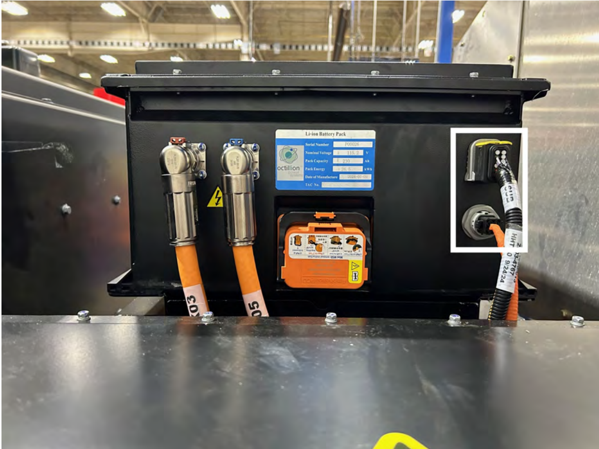
Figure 41. Communications Power Connectors (White Outlined Box)
