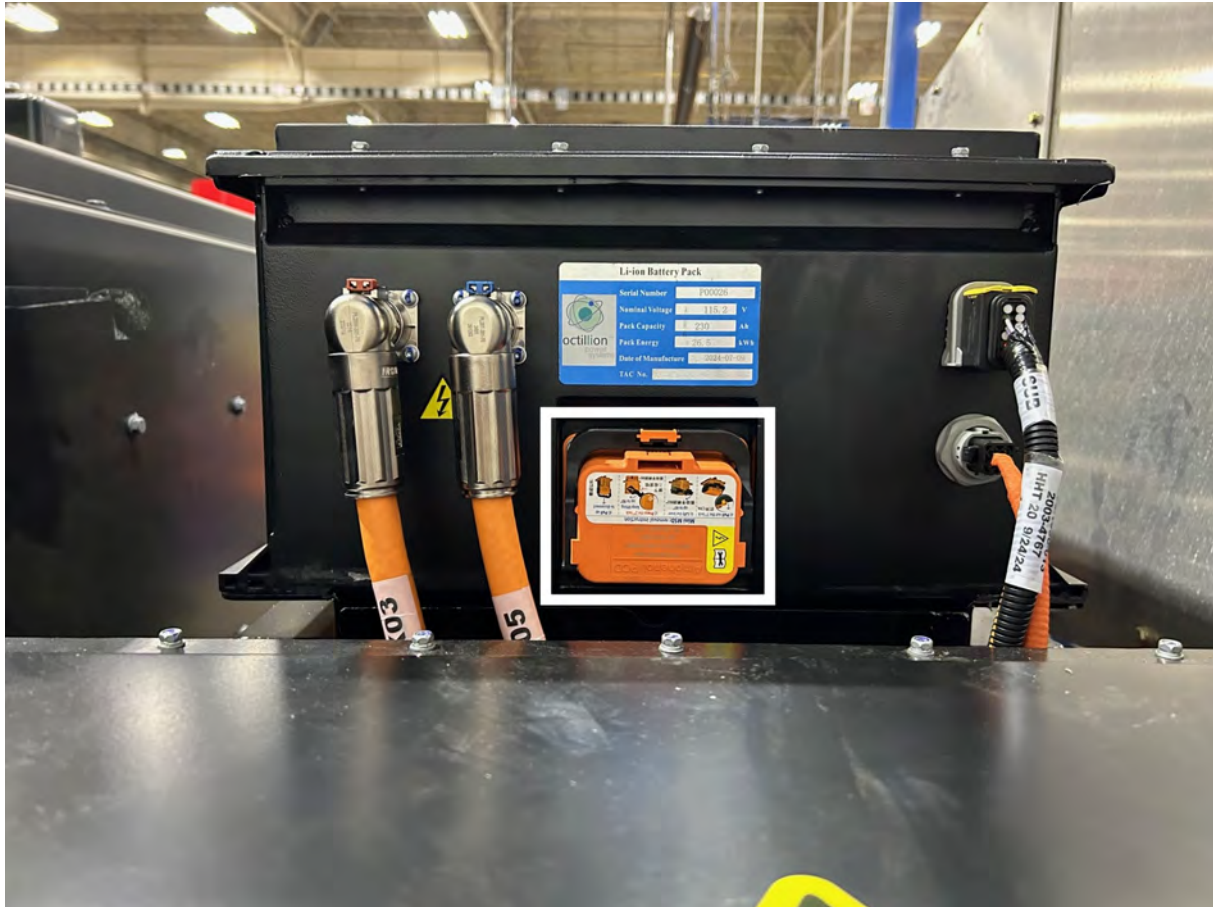
Figure 42. Main System Disconnect (MSD) (White Outlined Box)
