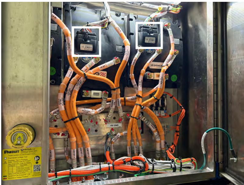
Figure 29. Body High Voltage Electrical Cabinet Panel 2 (2 Locations)
