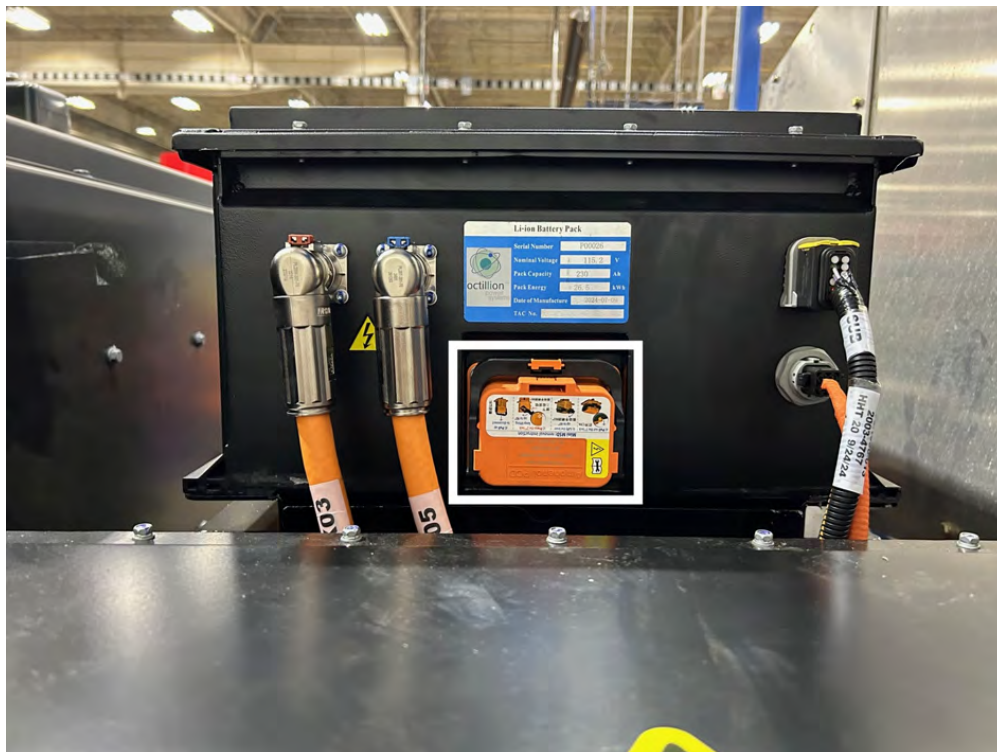
Figure 25. Main System Disconnect (MSD) (White Outlined Box)
