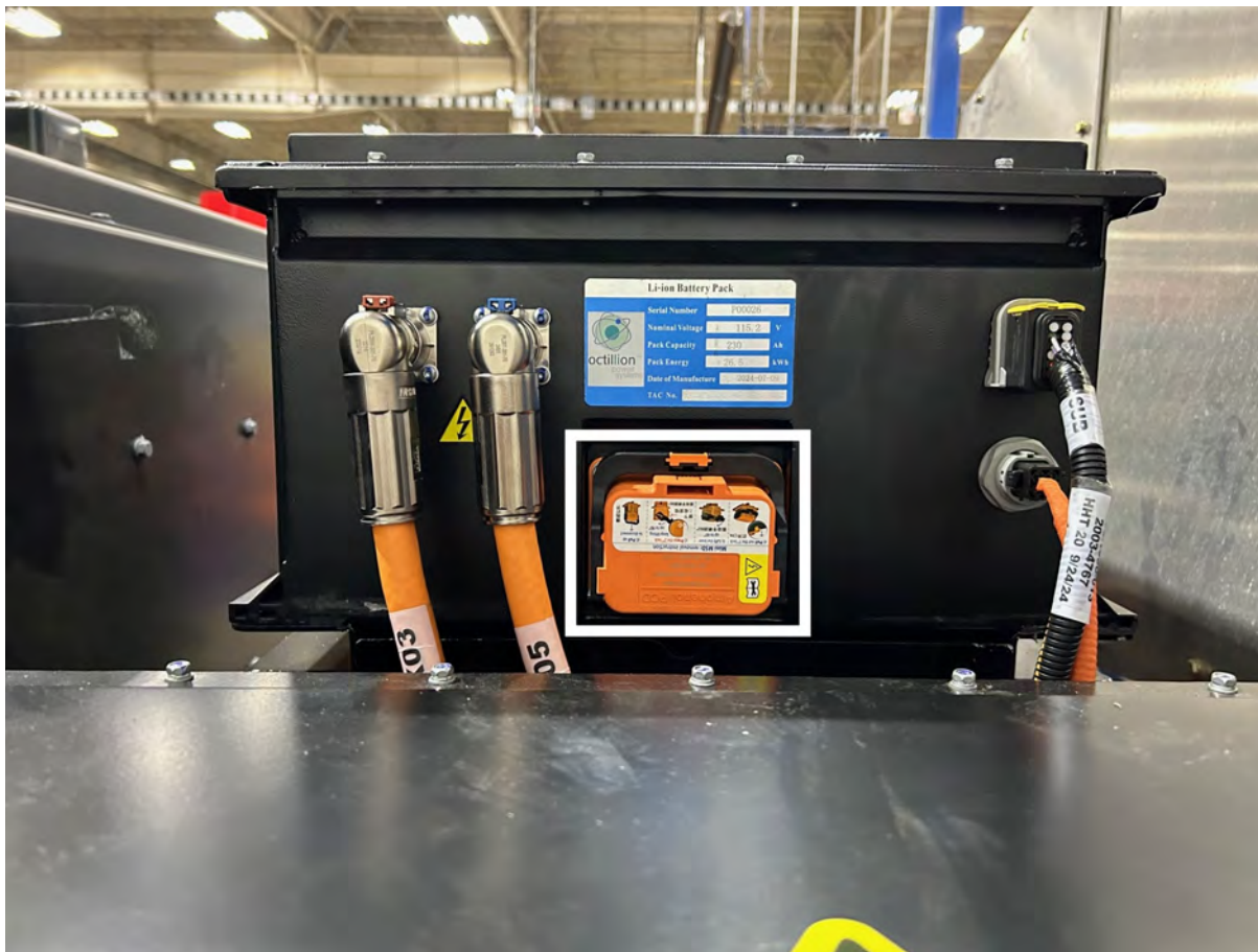
Figure 38. Main System Disconnect (MSD) (White Outlined Box)
