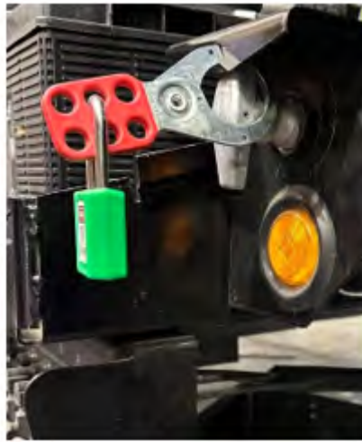
Figure 39. Chassis Battery Disconnect Switch
