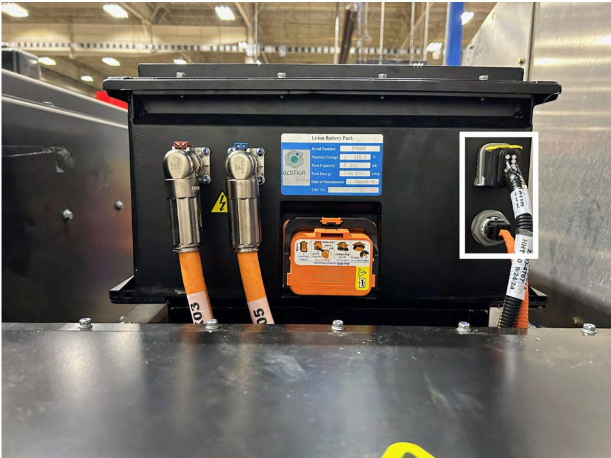
Figure 37. Communications Power Connectors (White Outlined Box)
