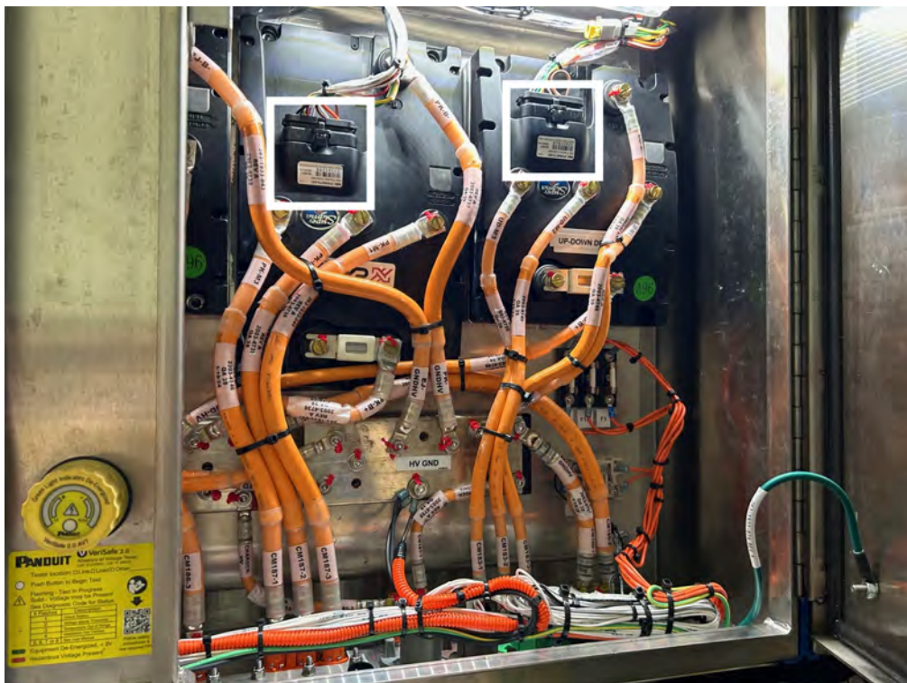
Figure 35. Body High Voltage Electrical Cabinet Panel 2 (2 Locations)
