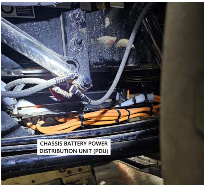
Figure 48. PDU Location on a Peterbilt EV Chassis Viewed from the Street Side Wheel Well Beneath the Cab
