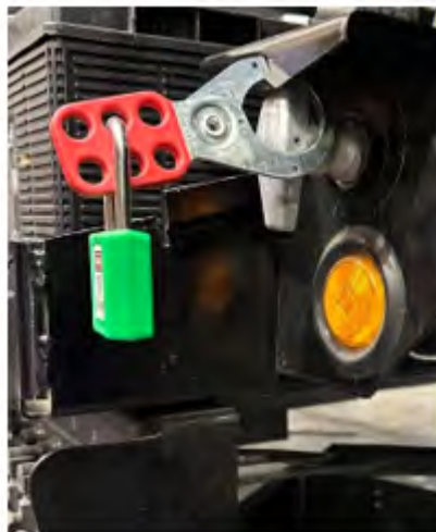
Figure 18. Chassis Battery Disconnect Switch
