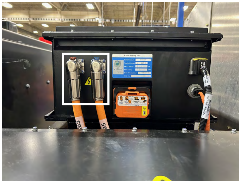
Figure 27. Battery High Voltage Power Connectors (White Outlined Box)
