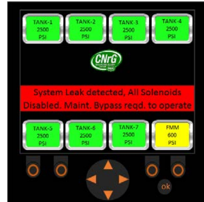
Figure 94. System Leak. Maintenance Bypass Required.
